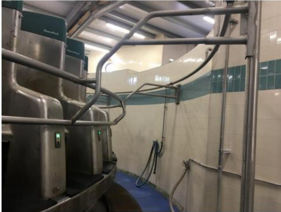
All of the walls in the milking parlour were tiled to allow ease of cleaning and it was very decorative!
