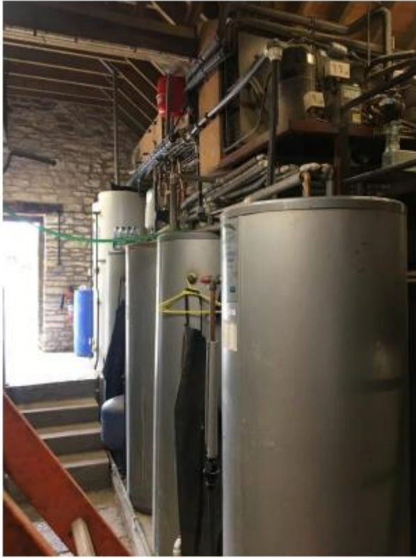
Vessels storing the water heated by the cooling compressors
