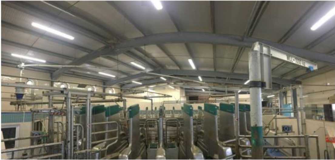
Deck Mounting/Dismounting area with gantry to remove robot units for service
