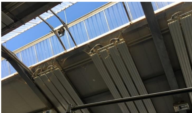
Fig 38. Automatic venting roof ridges and the heaters installed (currently oil heated but looking at wood chip heating)
