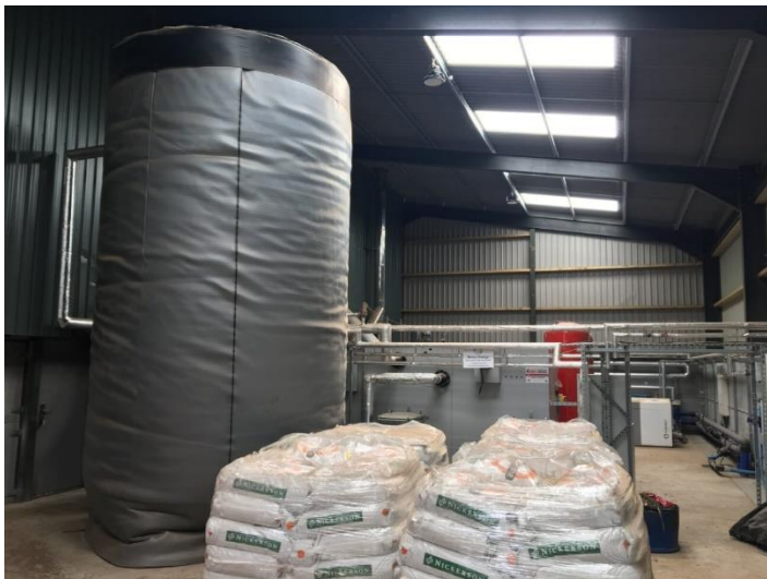
Fig 47. 800kW Biomass boiler
