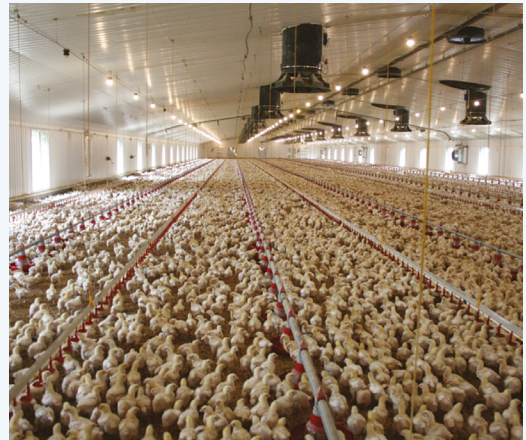
Ventilation inlets and exhausts mounted on the roof of a broiler shed.
