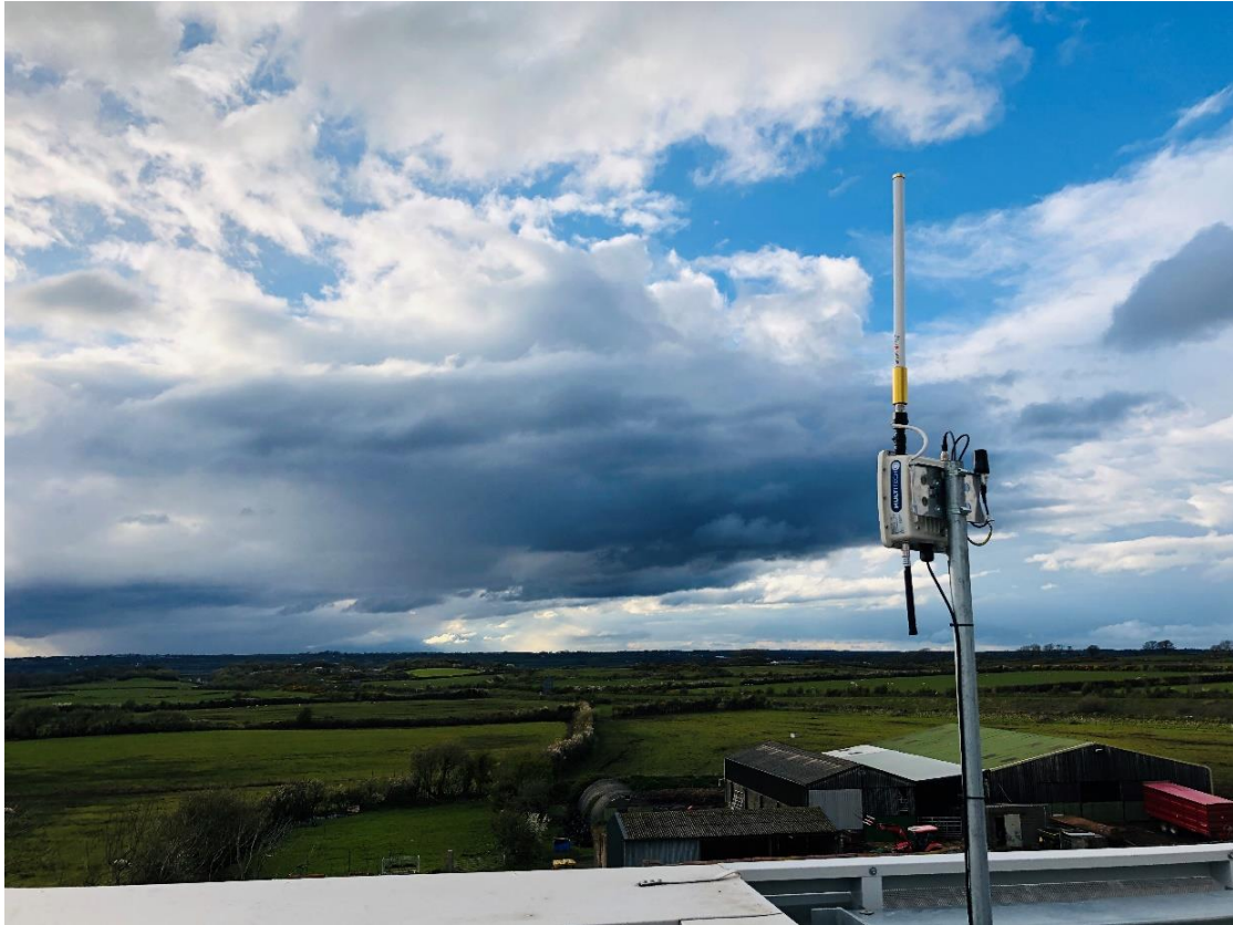
Figure 6: A 'MultiTech' gateway installed on the roof of the M-SParc Science Park near Gaerwen on Ynys Môn.
