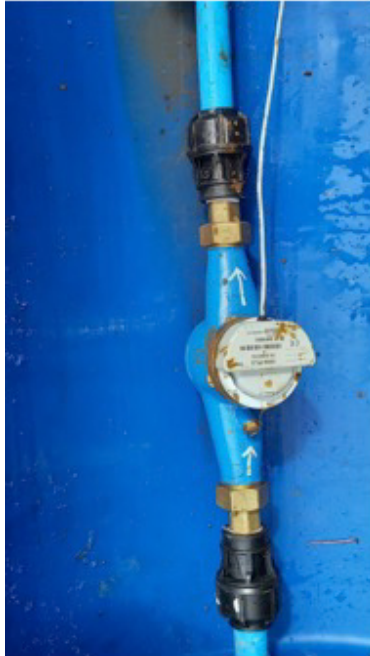
Figure 1. Inline water sensor
