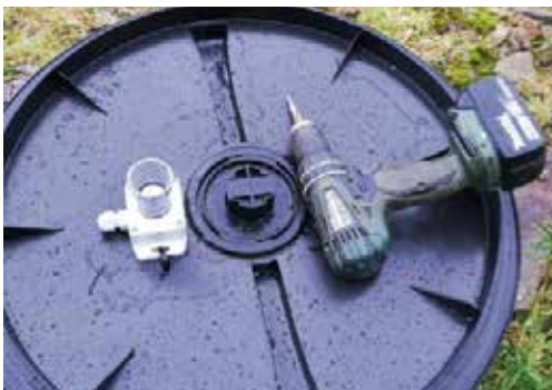
Figure 1: Fluid depth sensor installed on tank.
