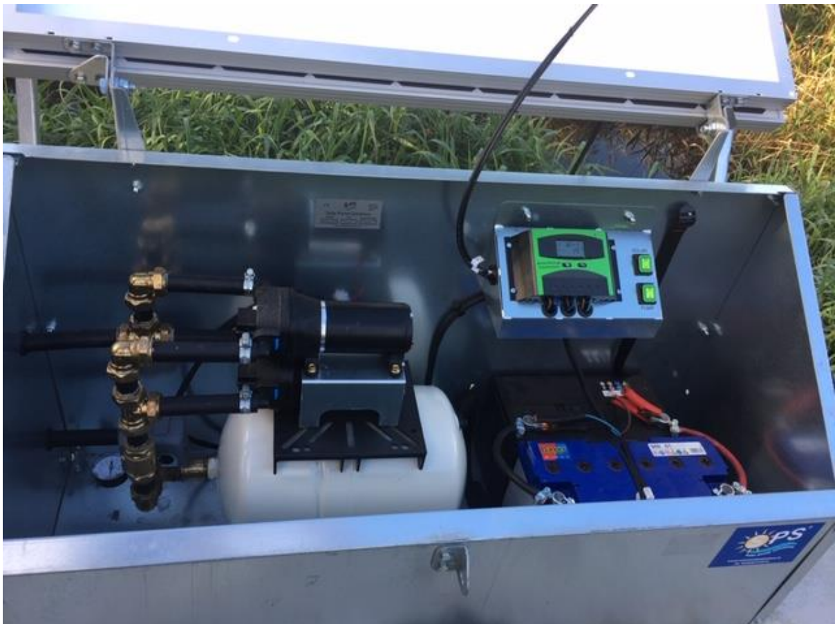
The solar powered water pump and electric fence set up that has revolutionised Pat Molloy's grazing and more than doubled his stocking rate.
