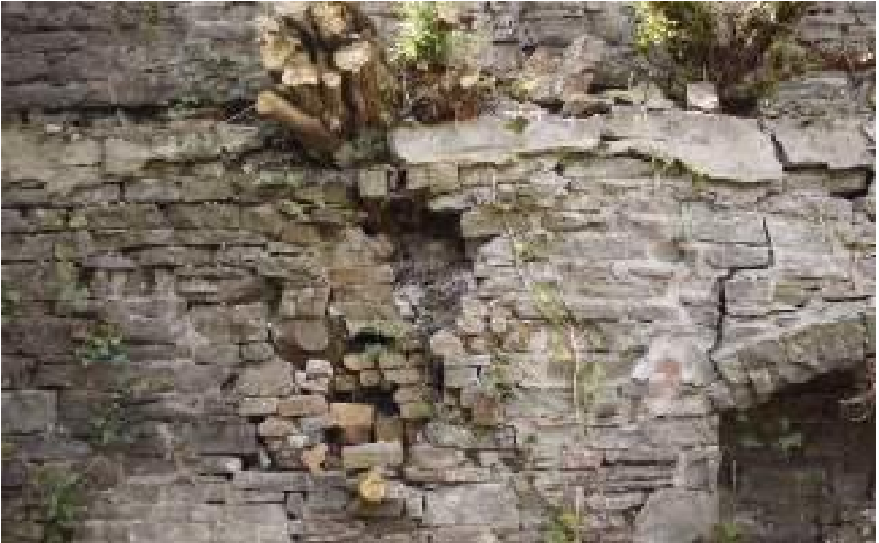
Illustration Four showing the poor condition of engine manufactory
