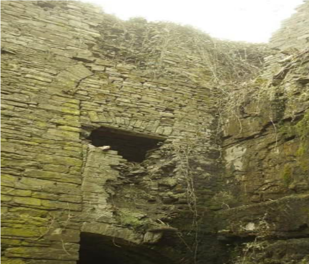
Illustration Three showing the dangerous structure of Furnace No.1.
