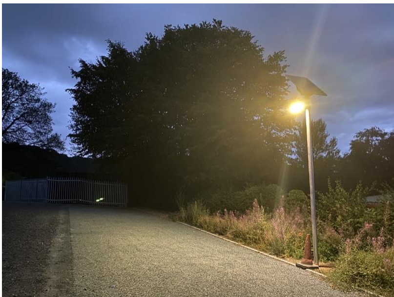
PV/solar lamps illuminating the pump track in Newtown.
