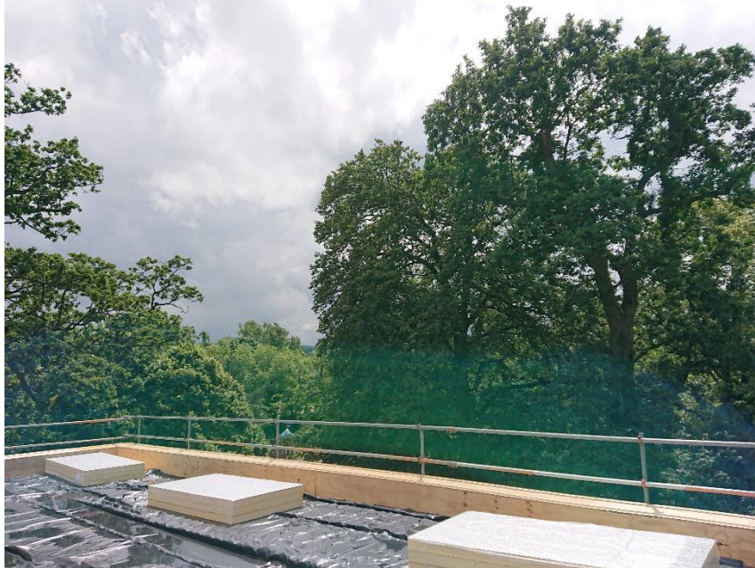
View facing south from the top of the new Riverside Venue building
