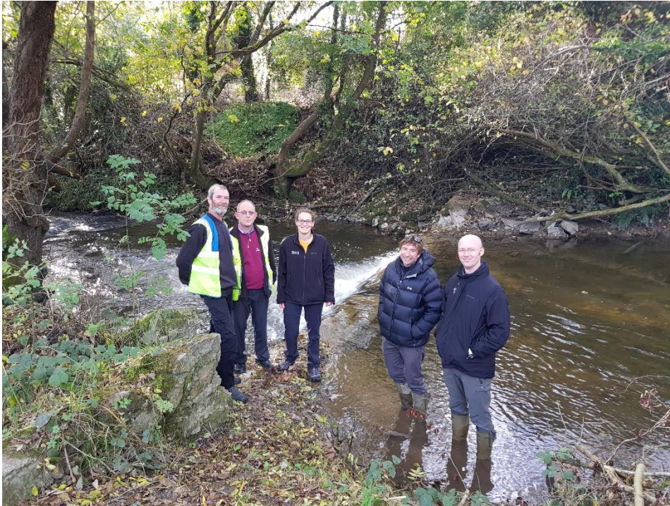
Stadco staff and Natural Resources Wales following successful partial weir removal on the river Cain
