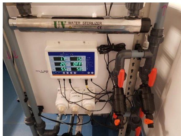
45 CEA controls unit
