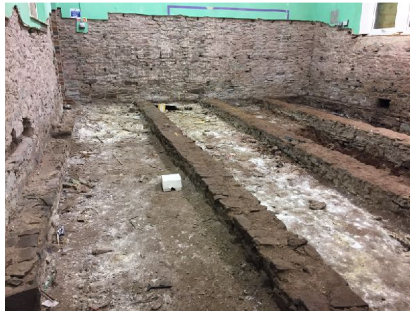
Floor structure and base of wall plaster removed in top eastern section.
