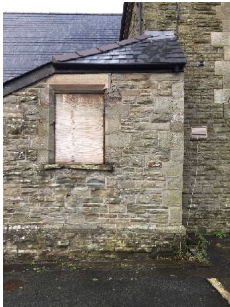
Southern frontage, separation of structure.
