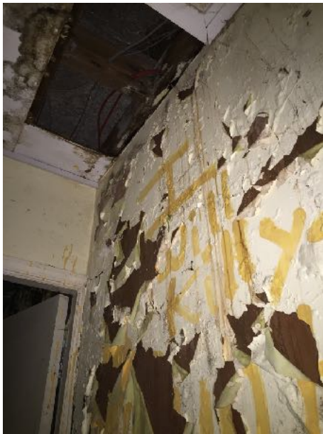
Water ingress at rear junction with ancillary structures.
