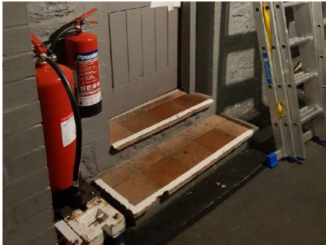
xR.1.06 - Steps to broken out to become stage level Accessible Dressing Room
