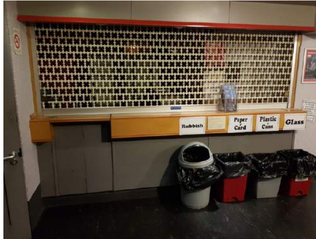
Existing Market Bar is too small and cannot operate all the times due to fire regulations
