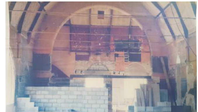
1978 - Castle Cinema - All partitions forming the modern rake are non original blockwork
