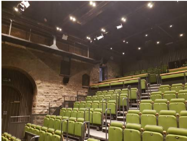
Market Theatre - lighting bridges. Replacement wire tension grid would create operational efficiencies for Tech team.
