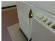
An example of un-insulated pipework
