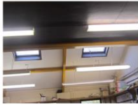
T8 lights with diffusers. Ideally, we would like to replace these with LED lights with reflectors
