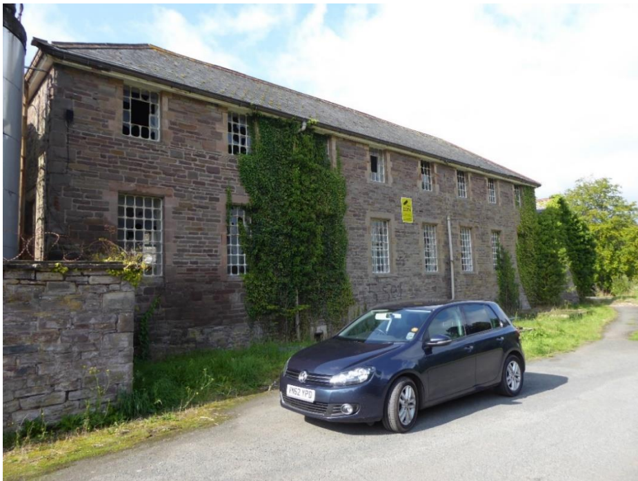
Fig 4 Former 2-storey workshop block to west of main block known as official block
